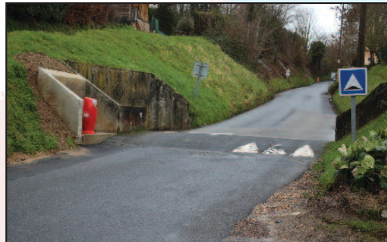
Borne incendie Route des 6 chemins
